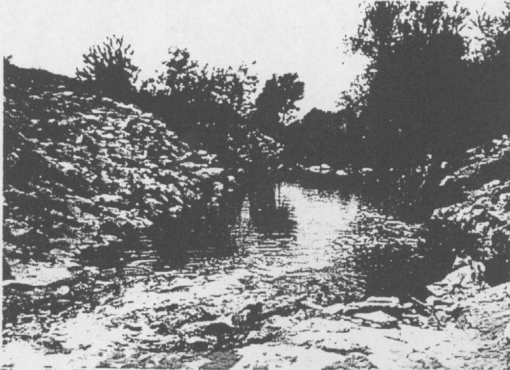
Photo #1: This photo shows the beginning of the restoration project area. Banks are steep (2:1 – 1:1) and unstable. Rip-rap has been used to stabilize areas.
